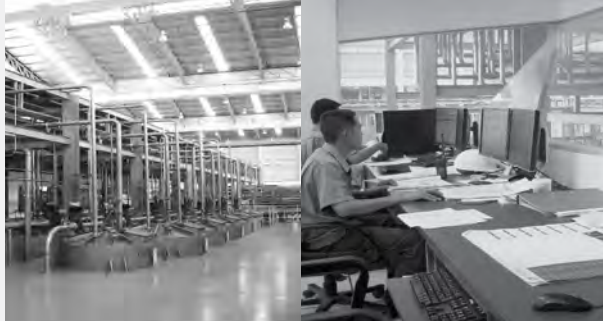
Loading raw materials for production through piping system by automatic control
